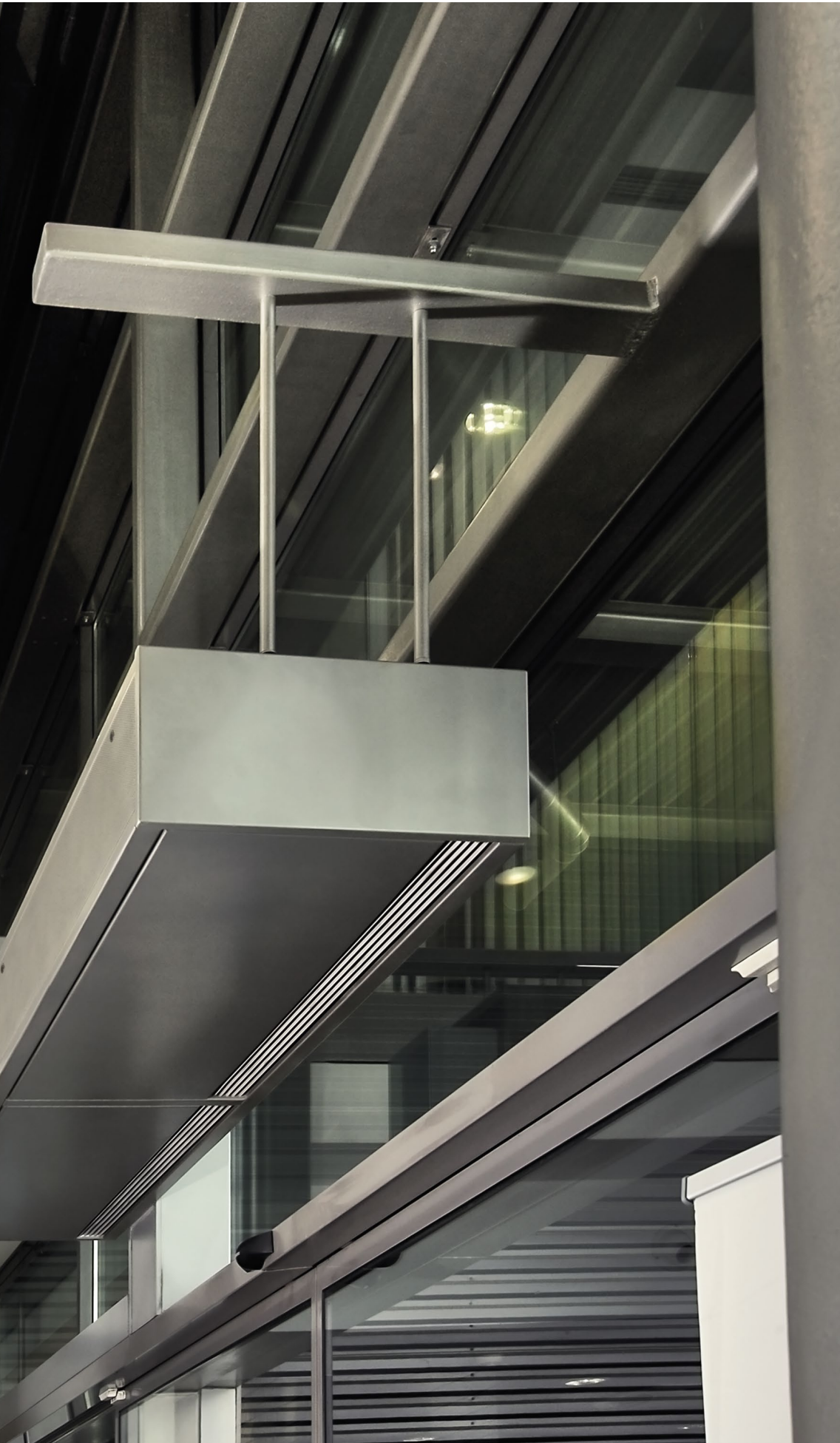
Porsche Centre, Moscow: The screening effect of UniLine door air curtains effectively counters heat losses and produces a comfortable interior climate.
